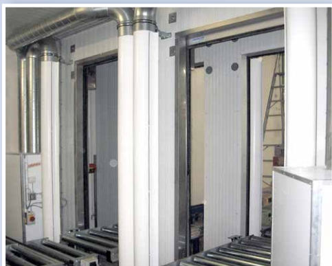
Conveyor doorways to Oxygen-reduced storage
