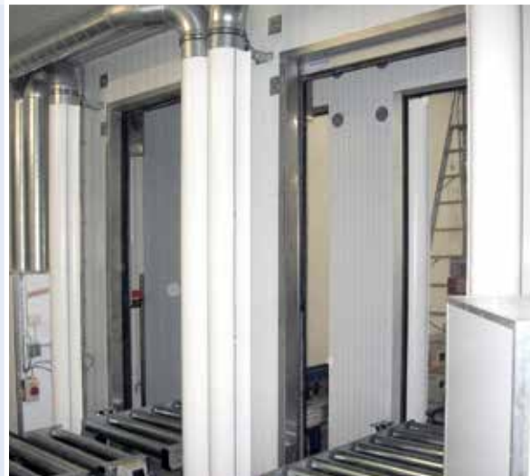
Coldstore logistic door for hypoxic air fire prevention
