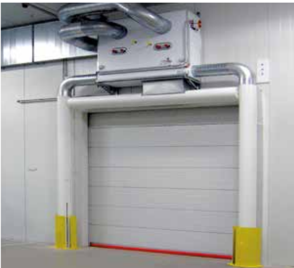
Coldstore logistics door
